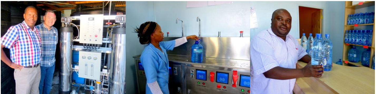
Left: Barrie Francis with businessman Anthony inspecting the water processing plant; Middle: the water is filtered again before it is dispensed. Right: customers can buy pure water in bottles or bring their own cans for filling.
